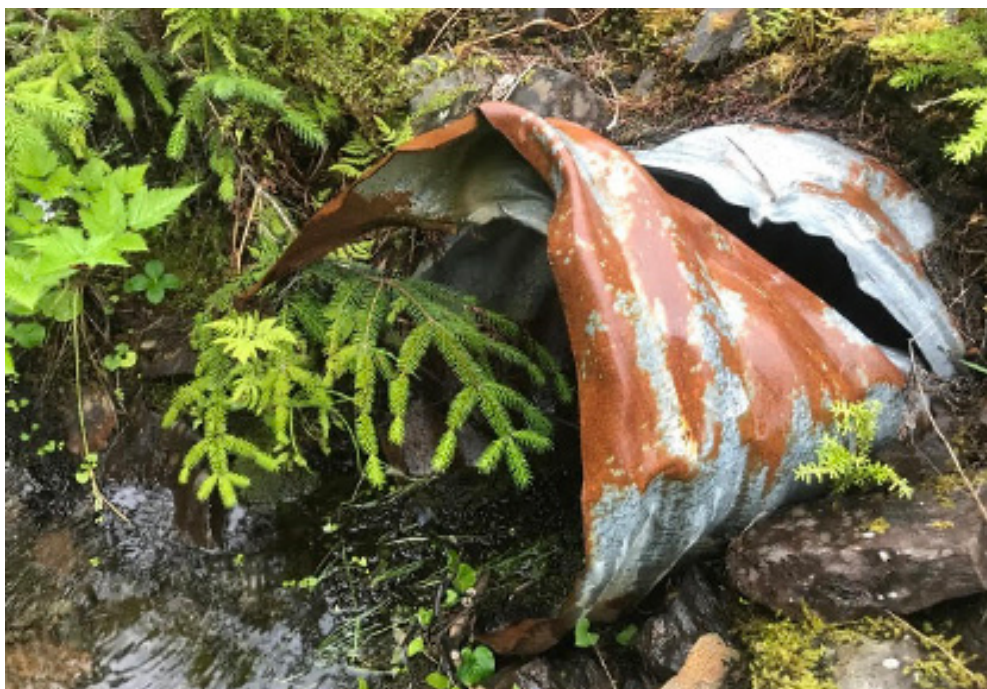
There are at least 447 failed culverts on Prince of Wales Island alone which the Forest Service is fixing at a slow rate of 5-6 per year. Photo credit: Alaska Sustainable Fisheries Trust.
